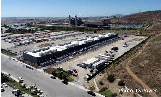
Gateway Energy Storage Project San Diego, California, USA 250MW for 1hr (250MWh) Li-ion Battery
